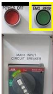
Figure 3-7: Controls in the lower area of the ISC cabinet
